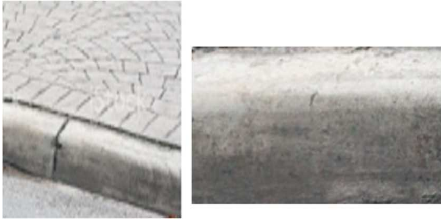
Fig. 4.22. Pattern 4. Real curb (Left), Example Pattern of 6 inches Wide, 6 inches Tall and 24 inches Long (Right)
