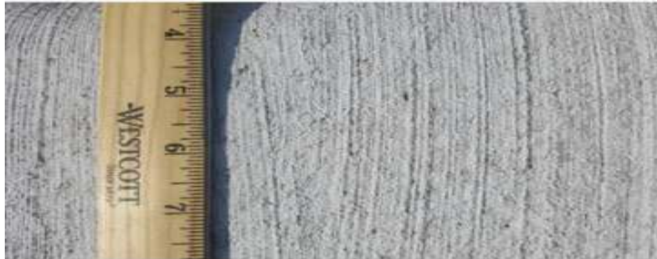
Fig. 3.8. The Surface of the Concrete Curb
