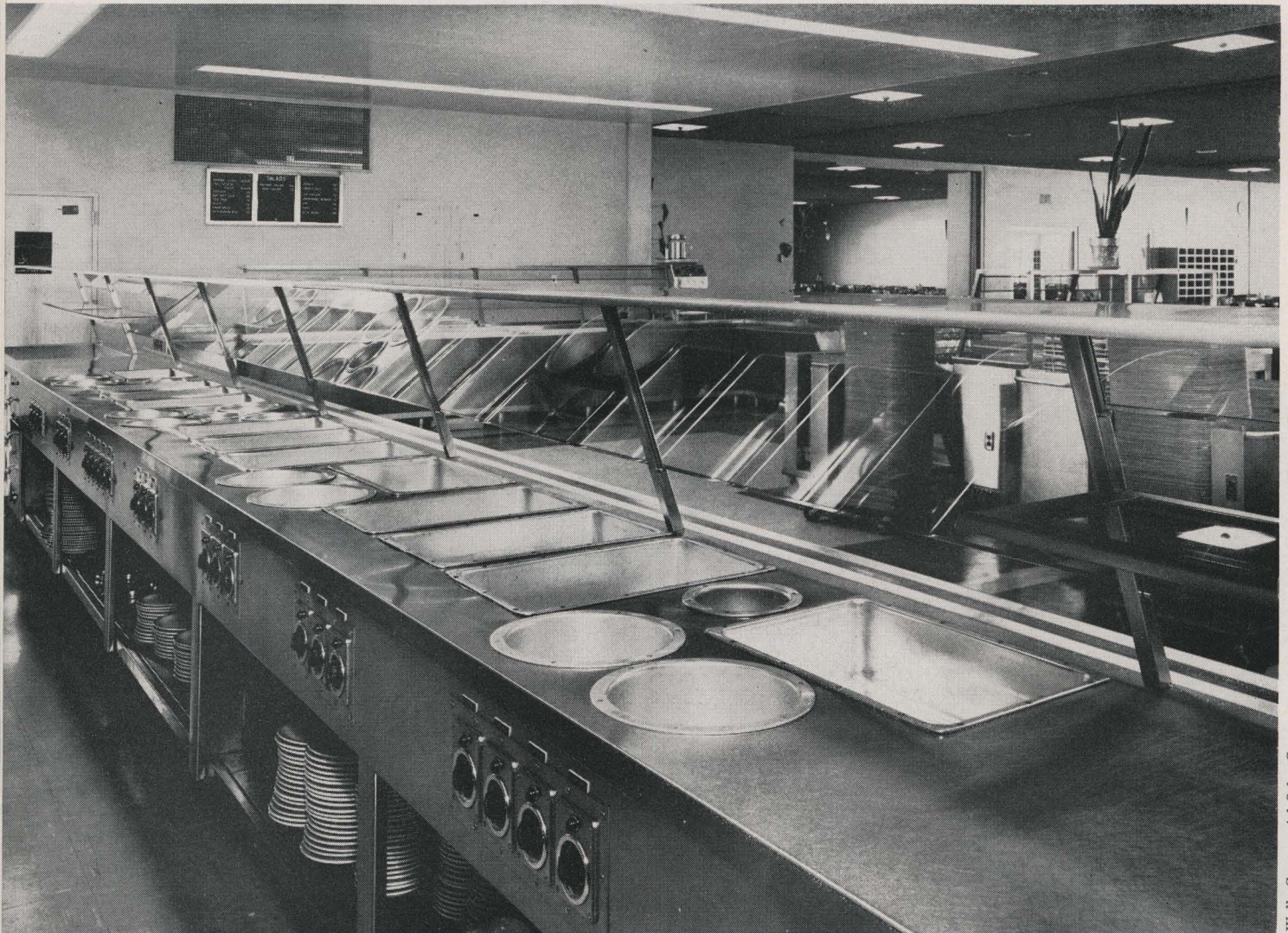
This modular, stainless steel electric cafeteria serving line has been designed for economy and speed.
