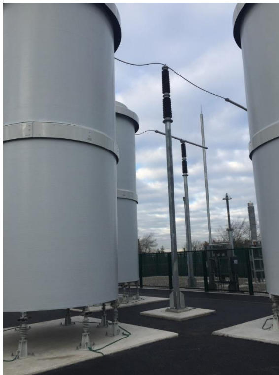
Figure 6.1: The 220 kV - 50 MVar Air Core Shunt Reactors.
