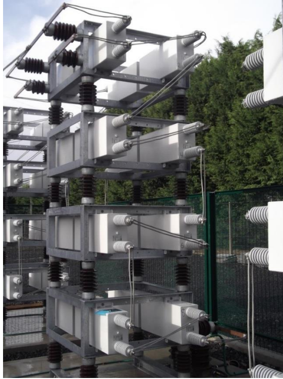
Figure 5.1: Shown is a 110 kV, 15 MVar Shunt Capacitor Bank.
