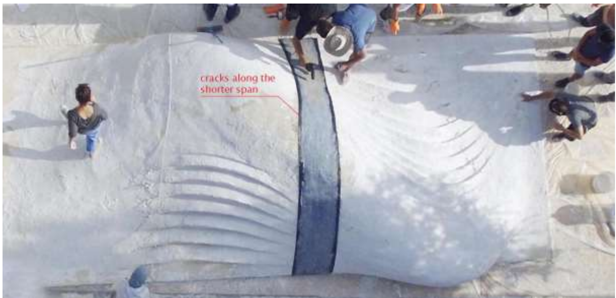
Fig.9: Cracks taking the same direction as the laying of the CCF Reference: Photographed by the authors - July 2018
