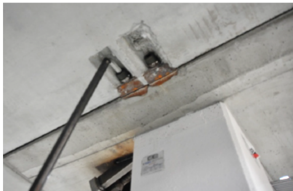
a) Activation of the loosen bolts to provide continuity to the longitudinal bars crossing the beam-column [6]
