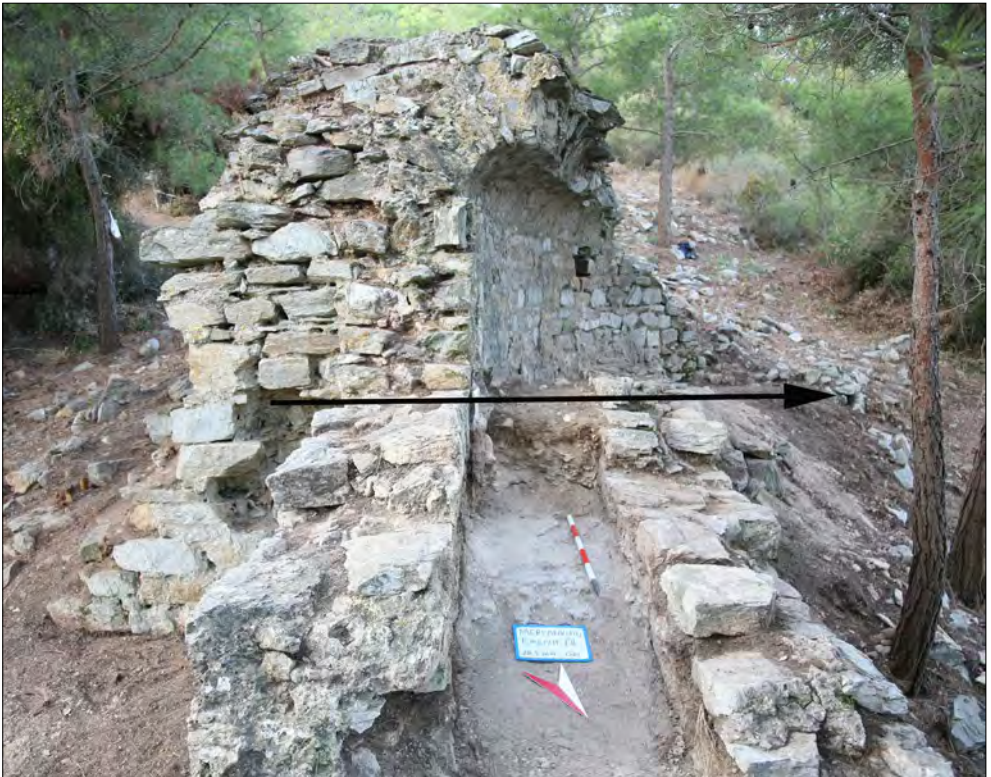
Fig. 21: Aqueduct at the beginning of the Mercankuyu Bridge: Hadrian channel below, vaulted corridor above the black line over which the Antonine channel was built.
