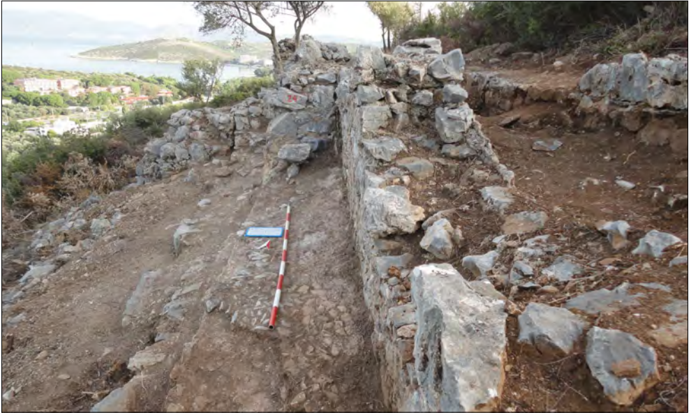
Fig. 24: Bypass line on the right, which uses the hillside wall of the then disused Antonine channel as valleyside wall for the bypass (with supporting pillar) in the middle and the Hadrian aqueduct on the far left (not visible).
