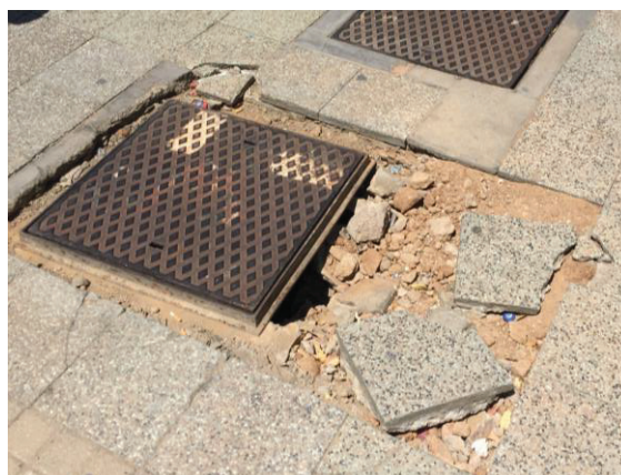
Figure 19 Damaged walkway on Independence Avenue (Source: Own photography)
