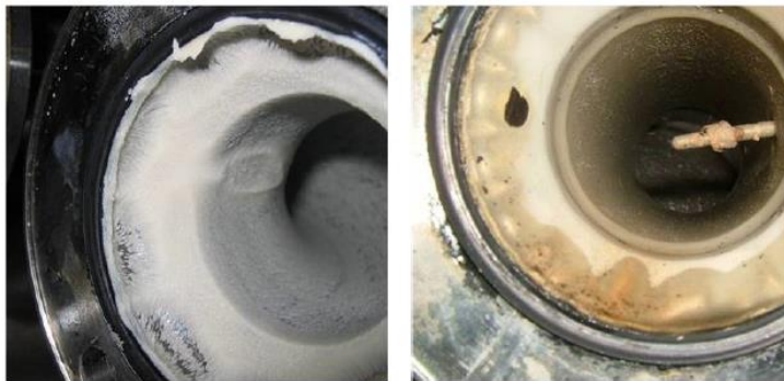
Fig. 2-13. Representation of protein fouling on the left and mineral fouling on the right.
