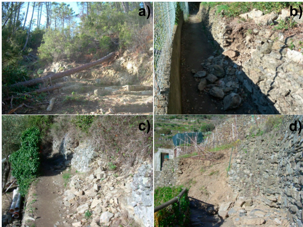
Figure 9. Examples of damage and/or rainfall-induced effects recorded using survey forms after a weather alert: (a) trees fall down; (b,c) small dry-stone wall collapses; and (d) dry-stone wall failure causing a local path interruption.
