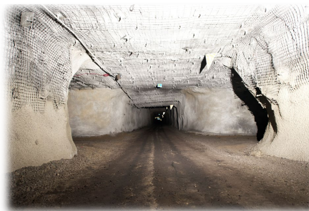
Figure 2: Underground Intersection rib support with FRS
