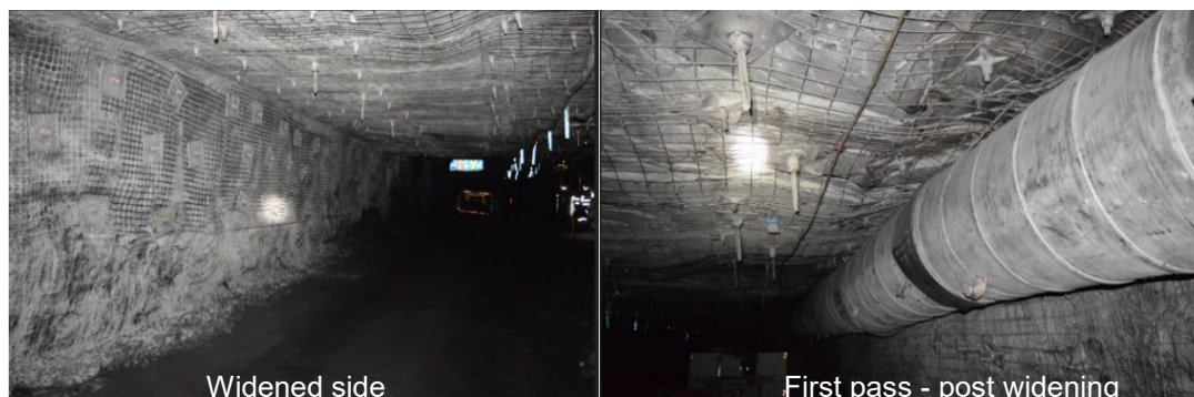
Figure 12: Second pass roof conditions and stress biased side deterioration of the first pass roof
