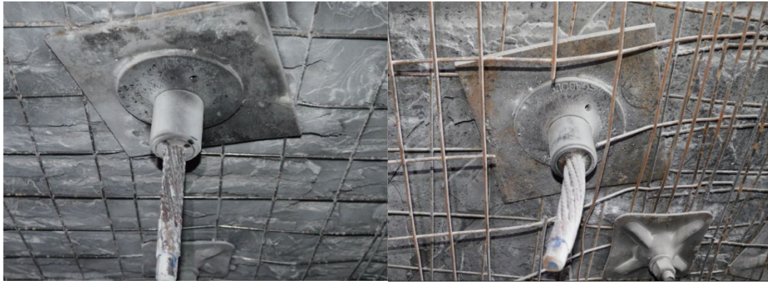
Figure 13: Collar loading on Jumbo cables
