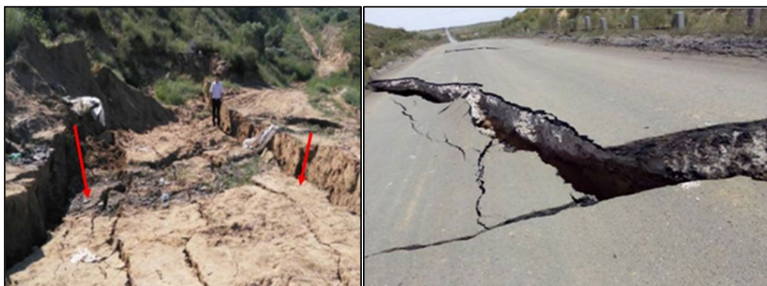
Figure 31. Bulianta LW22307 surface subsidence and cracking (Yang, 2019)
