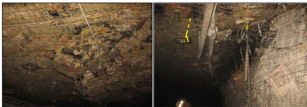
Figure 24. Austar gateroad centreline bagging and chain pillar side guttering near bent tendons (Moodie, 2011)
