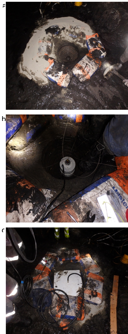
Figure 13: Installation of GEL floor extensometer (a: top of the hole reamed using auger, b: GEL extensometer placed into the hole, and c: steel plate covering the instrument)
