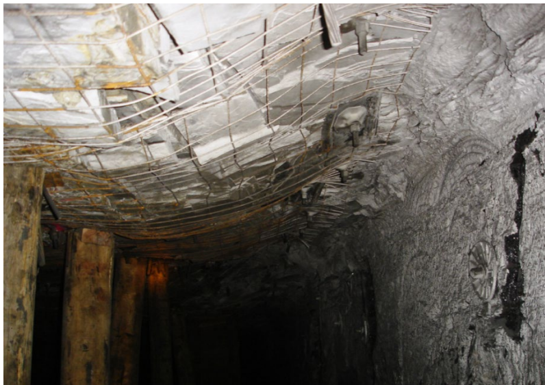
Figure 4: Example of guttering and roof sag requiring remedial support in 800 series
