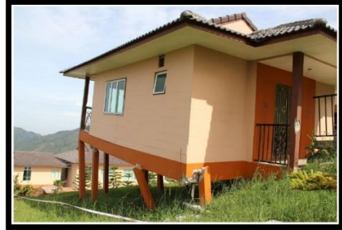
Figure 3. Properties damaged by the earthquake
