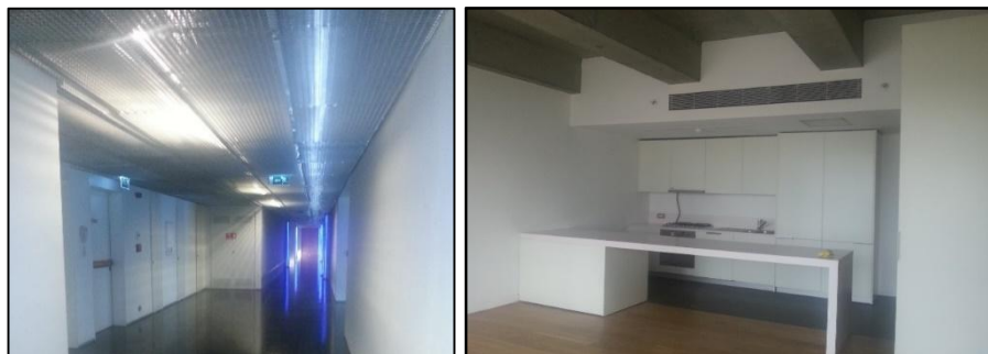
Figure 7.17: Suspended ceiling in the main corridors and the units of the Levent Loft1 project. Source: the researcher
