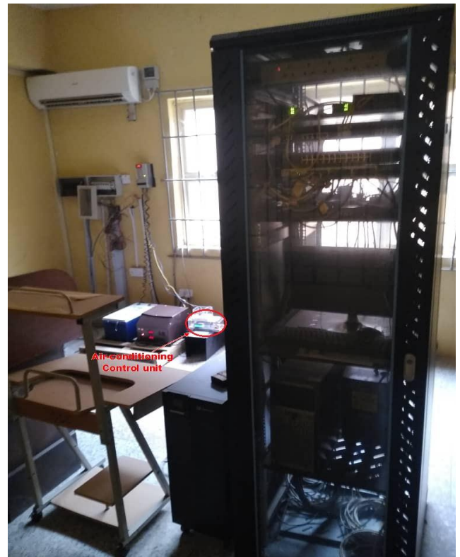
Fig. 7. The Server Room with the Deployed Air-conditioning Control Unit
