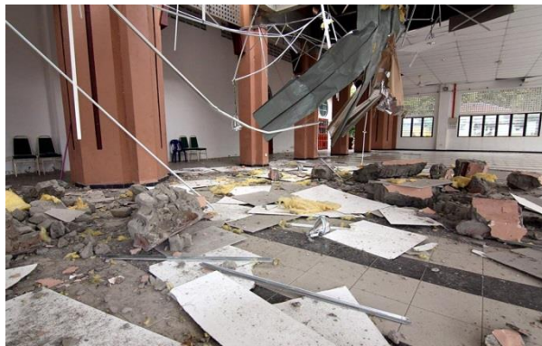
Figure 1.1 Damage during the Ranau Earthquake
