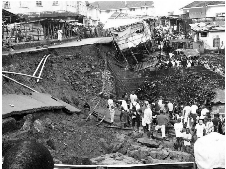
Fig. 1 Sierra Leone's King Jimmy bridge collapsed after torrential rains in August, 2013, killing 6 people.
