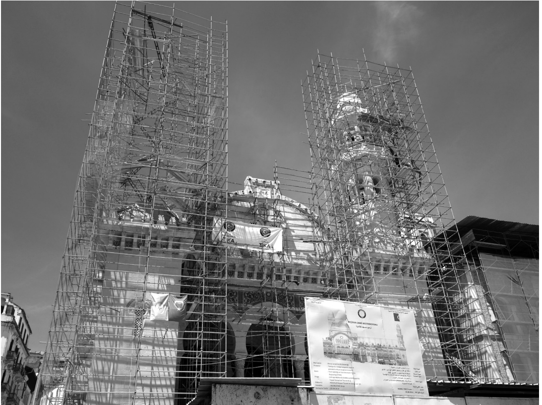
Figure 5.8 The Ketchaoua Mosque during the 2014–18 restoration funded by the Turkish government, Algiers. Photograph 2017. Source: Daniel E. Coslett.
