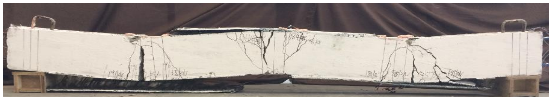
(d) Beams strengthened on both the hogging and the sagging moment regions (CB-C-F2-I40-TB)
