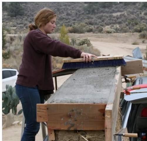
Figure 4.6: Roughed-Up Concrete Beam
