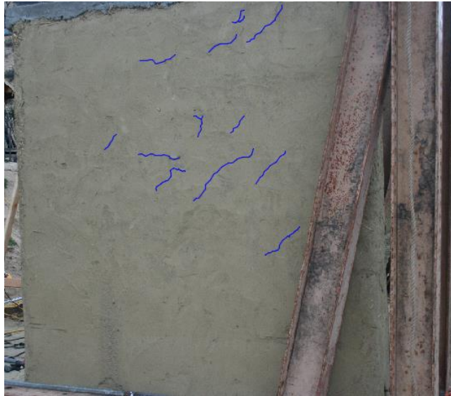
Figure 6.12: Wall Cracks at 0.5 inch Displacement
