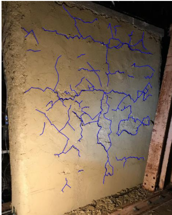
Figure 6.13: Wall Cracks at Failure
