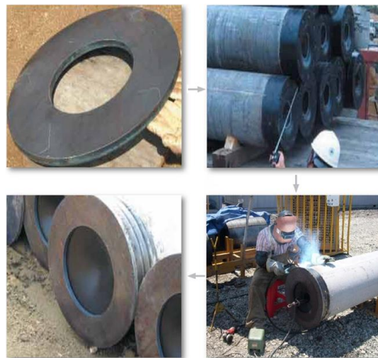
Figure 1. Ext composite pile: (a) extended steel plate; (b) pile dimension check; (c) welding connection; (d) Ext pile
