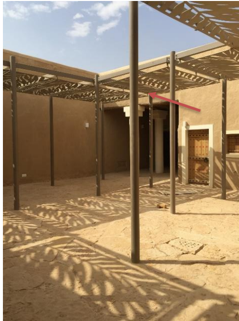
Figure 74: Addiriyah 1st Courtyard space – from January till February 2016 – cardboard was covering the metallic shed
