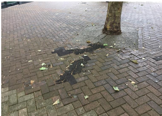
Picture 9: Poor repairs Abington Street Repairs need improving.
