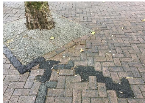
Picture 4: Poor repairs
