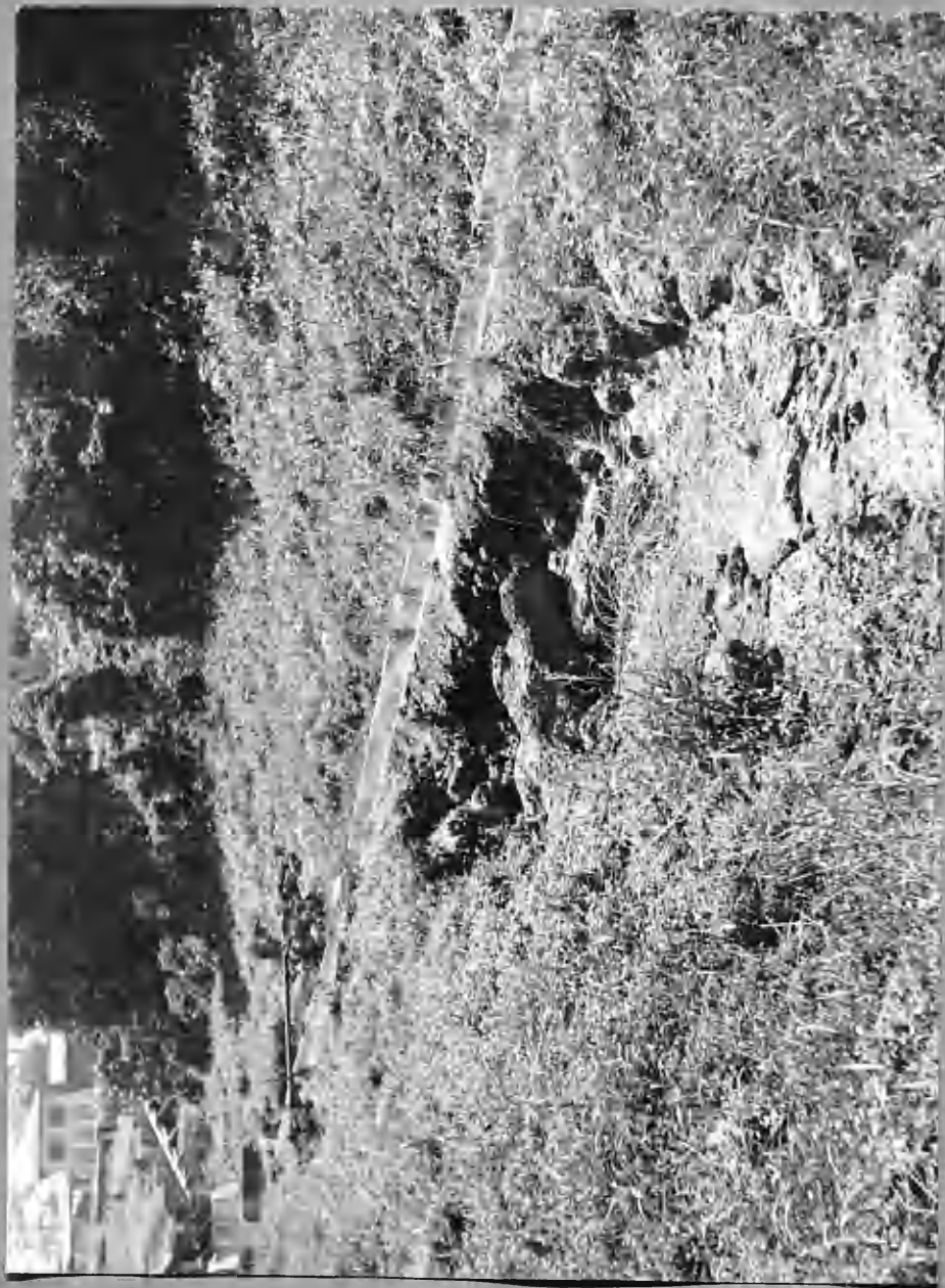
Photographs 9, 10 & 11 are of a concrete channel laid in 1942 in Preetown and smashed by heavy scouring.
