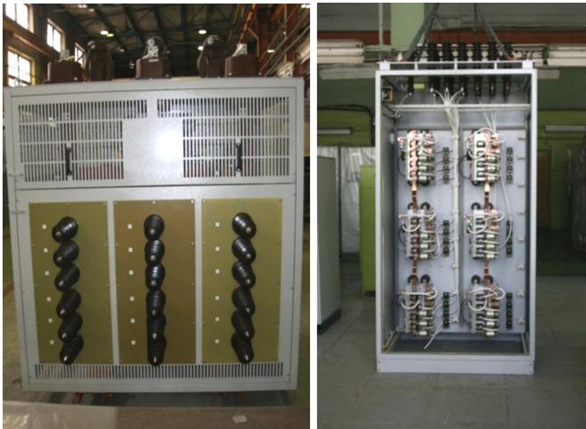
Fig. 4. Split windings transformer and rectifier unit at the distribution substation.
