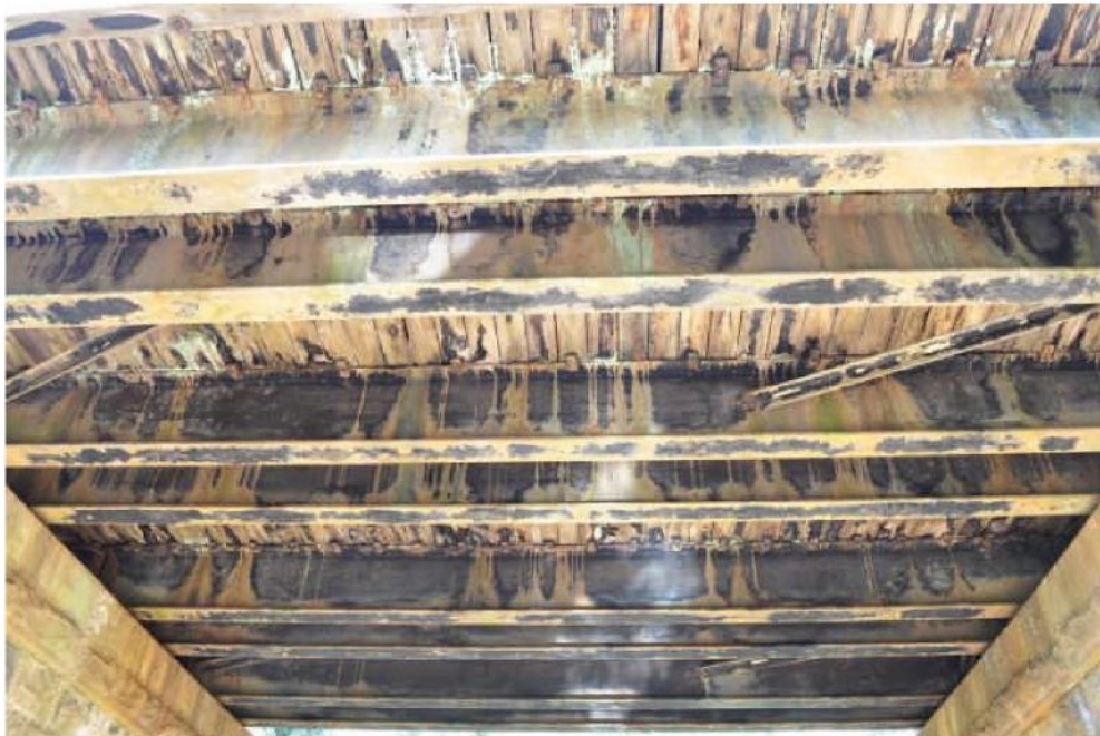
Figure 6 Surface corrosion of main girders of Bridge 62
