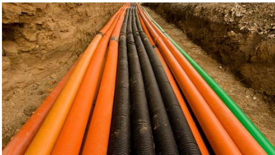
Buried inter building backbone cables
