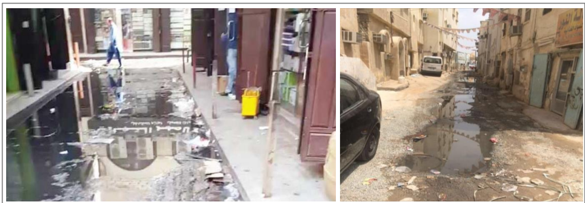
Figure 1-4: Sewer network problem in Jeddah’s historical area. Source right to left: Al-Fahmi (2016) on the and Salem (2017).
