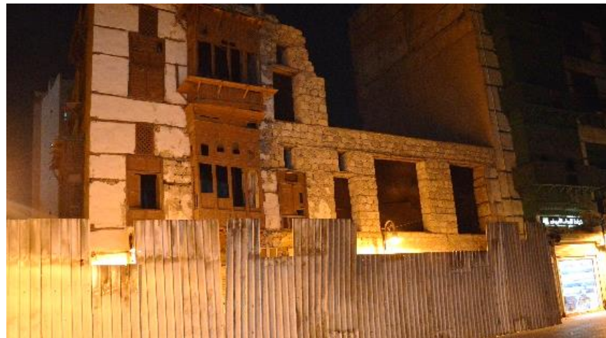
Figure 1-6: Neglect of Jeddah's heritage buildings. Source: Author contribution.
