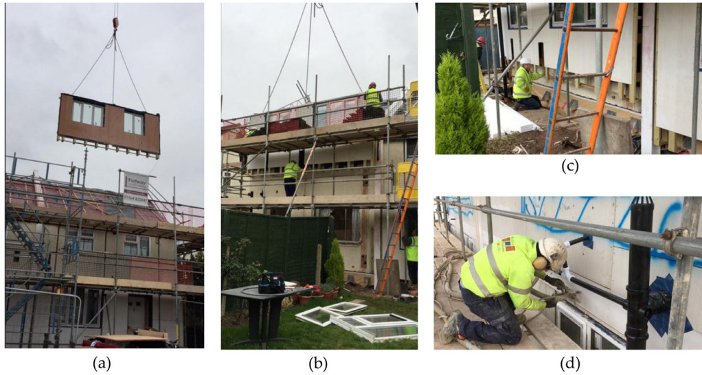
Fig. 8. Installation of the retrofit thermal envelope: (a), (b) and (c) – Stages of installation of an external prefabricated envelope panel; (d) Injection of thermal insulation into the installed external panel (source [7]).
