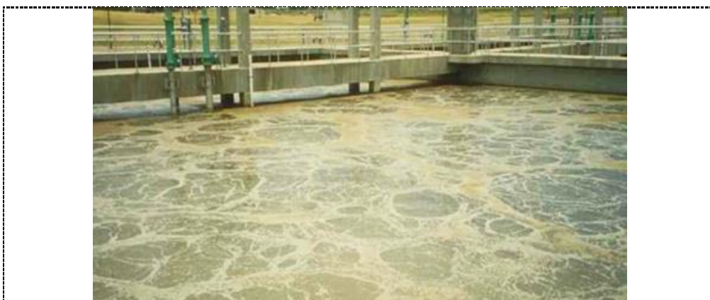
Figure 4. Aeration Tank in a typical WWTP
