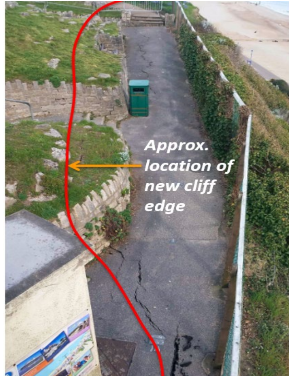
Figure 2 View of the public pathway leading to the beach front on top of the East Cliff, where the landslide incident took place in 2016. Red line denotes the new edge of the cliff after the incident.
