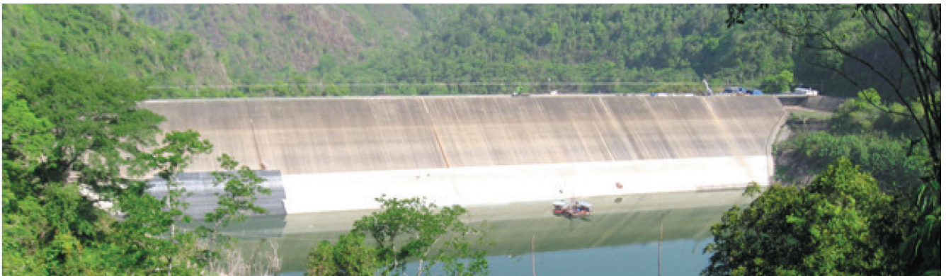
Fig.10. (Top) View of the upstream face of Turimiquire dam during the 1st campaign of the waterproofing works; (bottom left) the downstream face before the waterproofing works and (bottom right) after the waterproofing works
