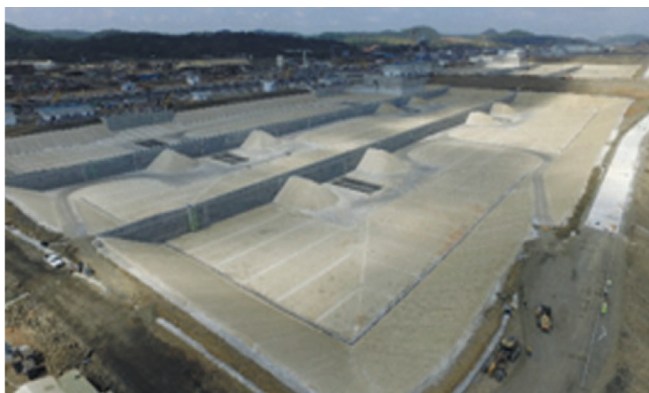
Fig.6. Aerial view of the Basins at the Pacific side upon completion of the waterproofing works
