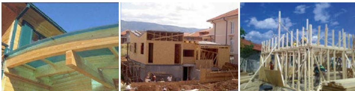
Figure 31: Wooden constructions: laminated wood (Bulart) (left), and timber buildings under construction (middle and right)
