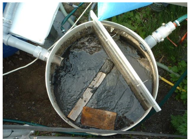
Photo A8: Excessive sludge accumulated in ST.
