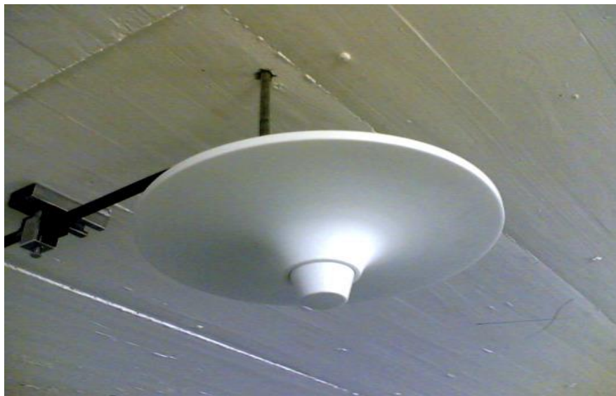
Figure (3): Pico cell base station
