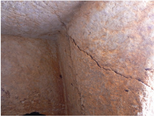
FIG. 21 Cracks in the main chamber of Tomb 2. (Photo courtesy of the authors.)
