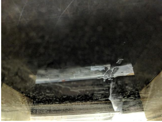
Figure 6.2.1: Water penetrating the flooring seam (seen from below the acrylic testing apparatus)
