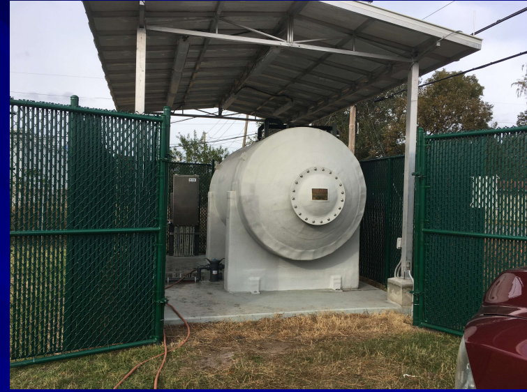
Alum Storage Tank
