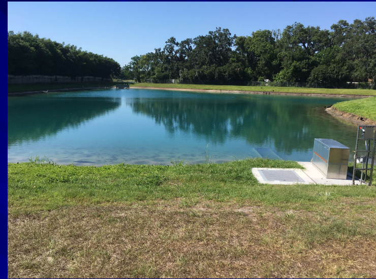
Water recirculation pump
