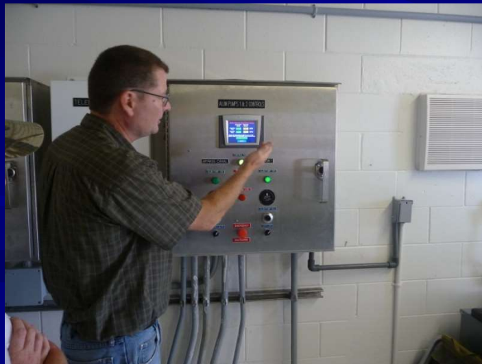
PLC Pump and System Controller
