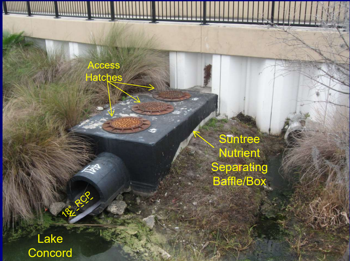
Exterior of the Lake Concord Suntree Baffle Box
