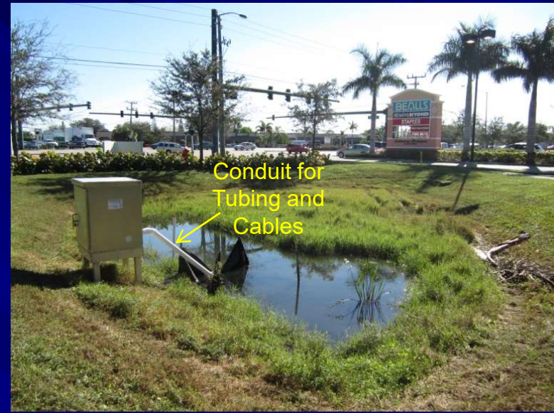
Site 1 – Pond 1 inflow monitoring equipment
