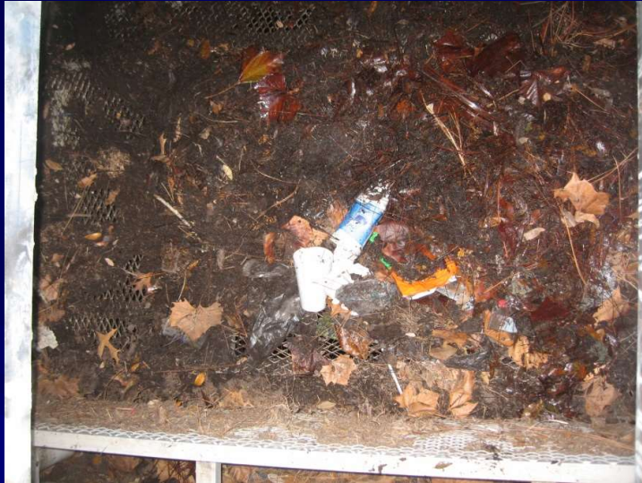
a. Accumulated vegetation on the screens
