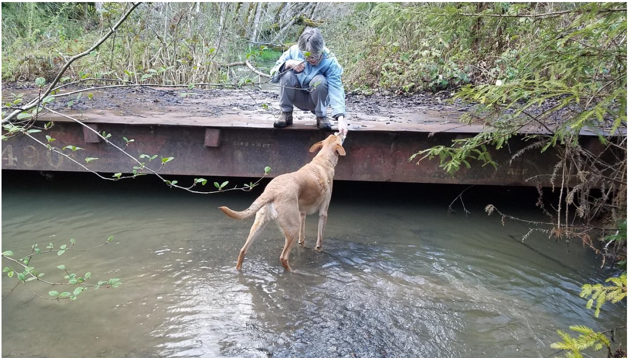
Figure 4: Aggradation of the Hall Creek channel can be seen in this picture of the railroad car bridge across Hall Creek. There is little clearance from the gravel bar in the center of the stream to the bottom of the bridge. The creek has become noticeably shallower here in recent years (McAdams, personal communication, 2018). Photo by Ethan Luckens.
