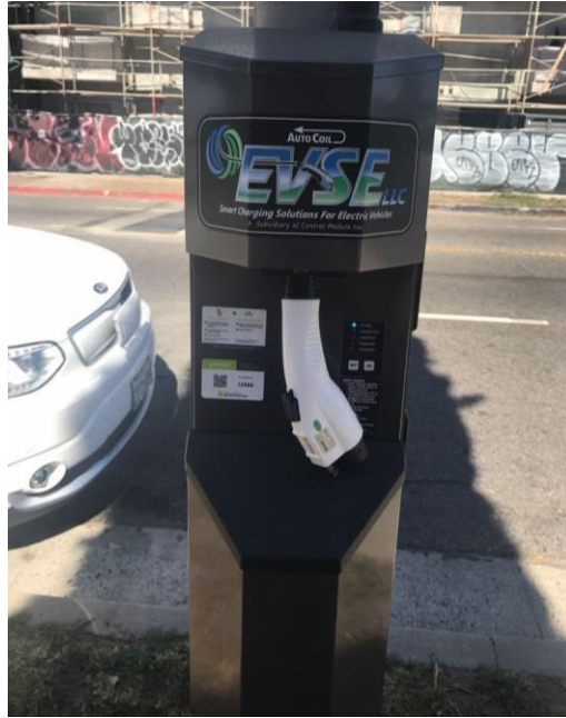
Figure 4-3 Close up view of public electric vehicle supply equipment located at 932 S Wilton Pl., Los Angeles. Image from PlugShare.com.
