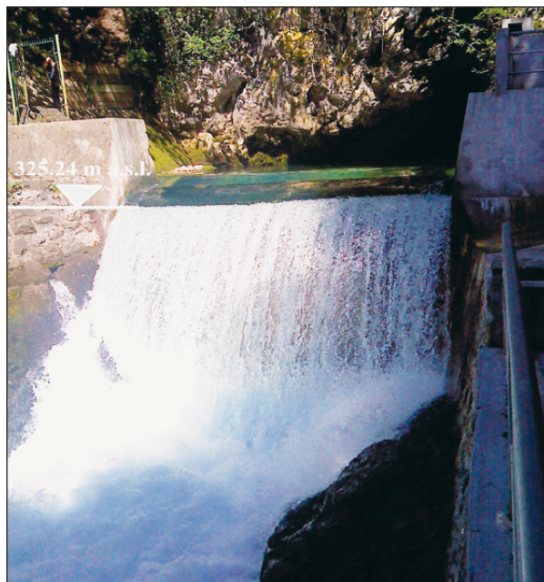
Fig. 5: The dam constructed at the exit of the Rječina spring cave (Photo: VIK Rijeka).
