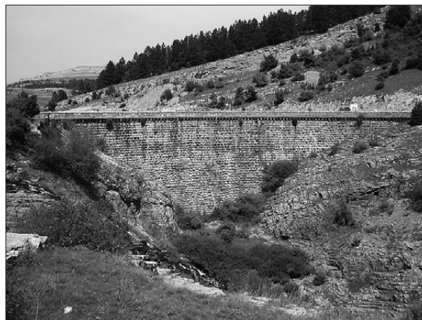
Fig. 6: Klinje dam. Still functioning successfully (Photo: P. Milanović).
