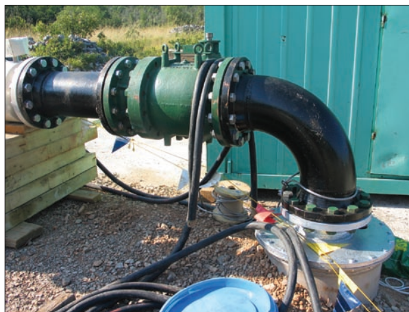
Fig. 3: Well B-10/06 connected to temporary pipeline (Photo: K. Mezga).
