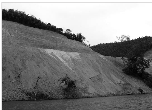
Fig. 21: Major new road construction alongside the Nam Ou near Muang Khua, involving large volumes of sediment being displaced into the river channel (Photo: K. Kiernan).
