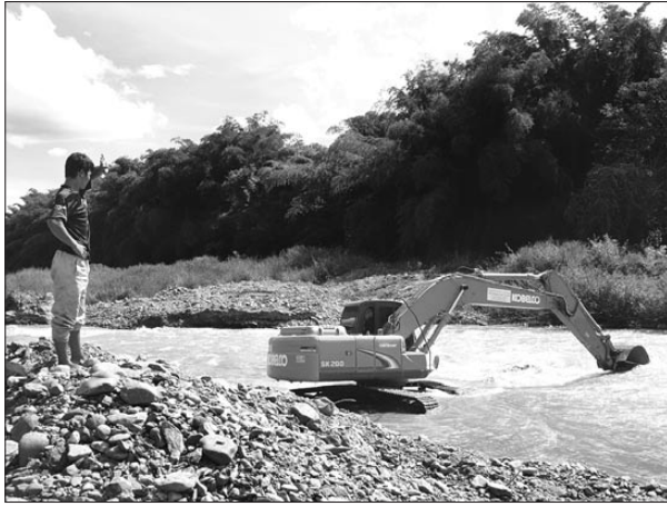
Fig. 19: Larger scale, mechanised alluvial gold mining entails greater disturbance of channel beds and release of sediment plumes. Here a commercial boat operator delayed by channel derangement negotiates with a mechanised alluvial gold miner to re-open the navigable channel to allow his own enterprise to continue (Photo: K. Kiernan).
