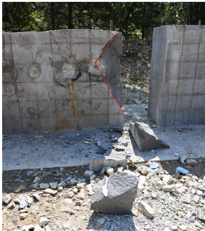
Figure 4.12. 50 psi seal failure plane symmetry
