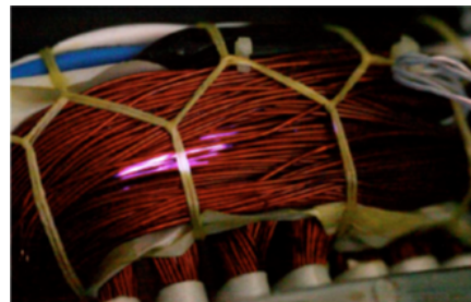
Fig. 1. A typical phase-to-phase insulation failure [4].
