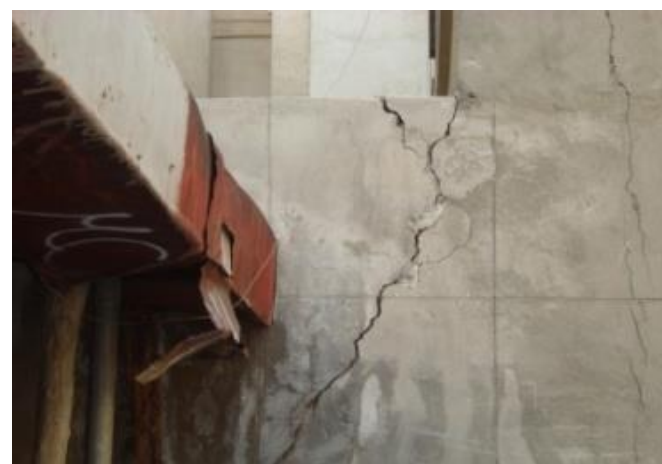
Figure 3. Cracks on wall of garage near the mentioned building
