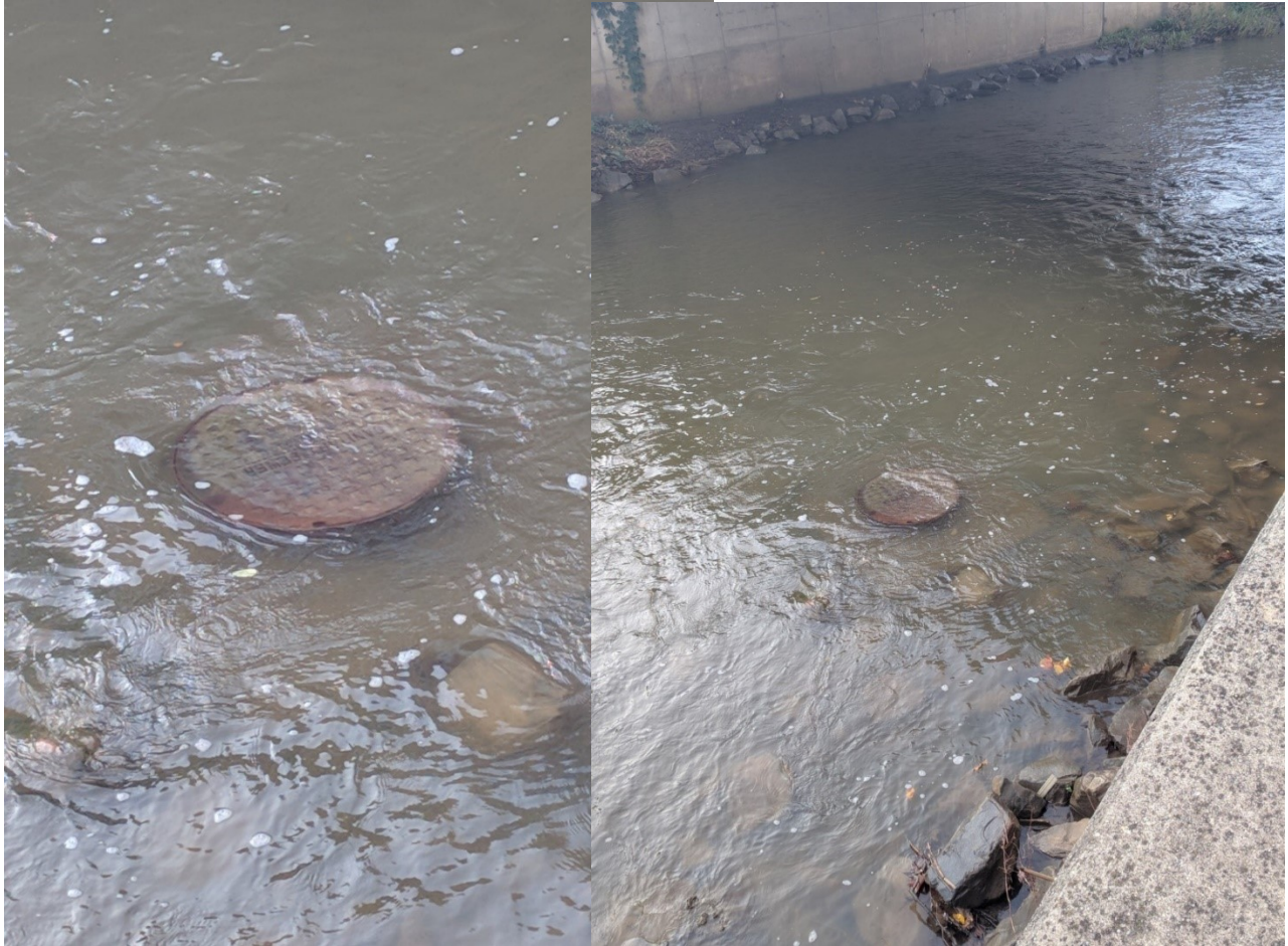
Figure 41. Sewer manhole covers with Pine Creek flowing over them at high flow situations.
