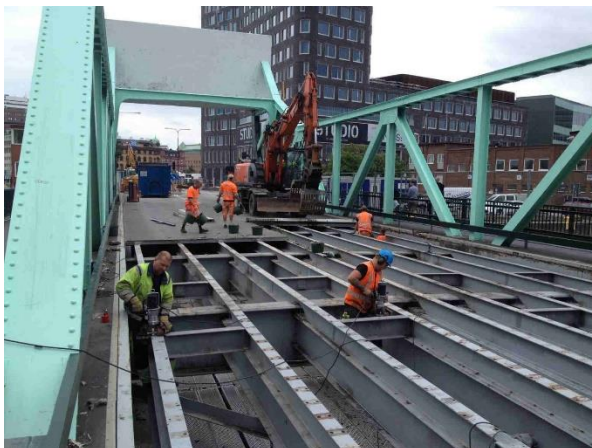
Figure 5. Removal of the old steel deck and preparation of the stringers for installation of FRP panels, Photo courtesy of Per Andersson
