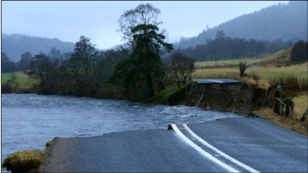
Figure 7.14. Damage to A93 road connecting the villages Ballater and Braemar. Source: BBC, 2016c.
