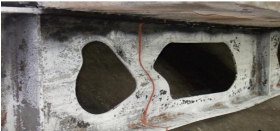
a) Deformed beam 2, experiment
