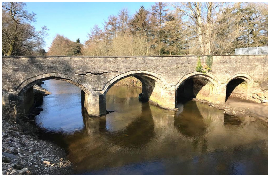
Figure 1. Scour at the front of the central pier led to scour-induced failure of failure of an arch bridge (Ballynameen Bridge) over the River Faughn near Cladys, Northern Ireland. (View looking from upstream of the bridge)
