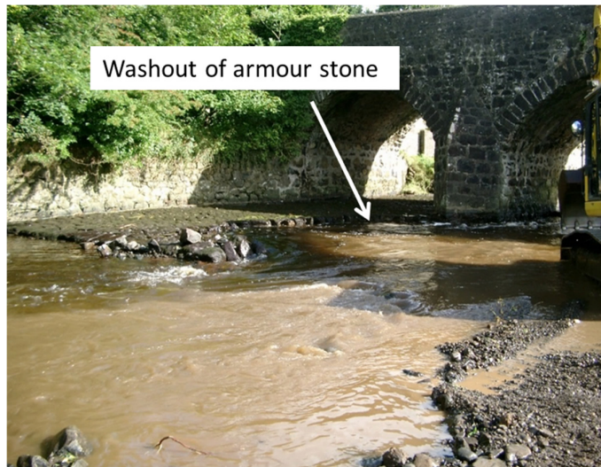
Figure 8. Supercritical flow immediately downstream of this arch bridge washed out armour stone placed there, and then (via a head-cutting mode) eroded the downstream bed; Co. Antrim, Northern Ireland
